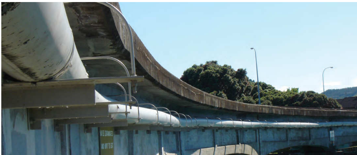
Support brackets for Poliplex® pipe including allowance for expansion and contraction.
